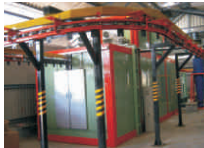
A view of the new conveyorised powder coating plant
